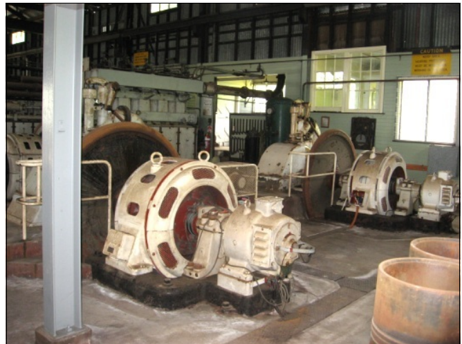
A recent photo of the two original GEC alternators with exciters. The two turbines are partially hidden behind the big flywheels. G. Estcourt.
