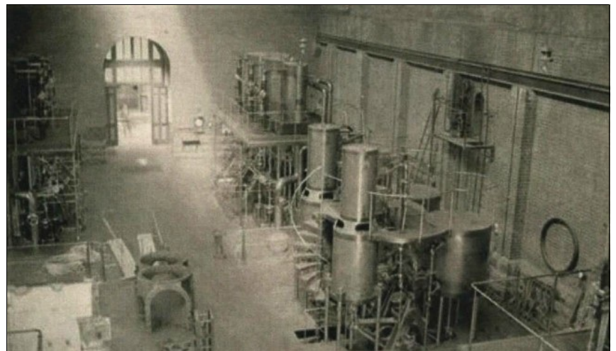
Three generations of steam pumping engines in the South Engine House at Spotswood At right, an original Thompson engine – rear & centre, the Hathorn Davey engine – left, the Austral Otis engine to an E.P. Ellis design. Image courtesy Museum Victoria
