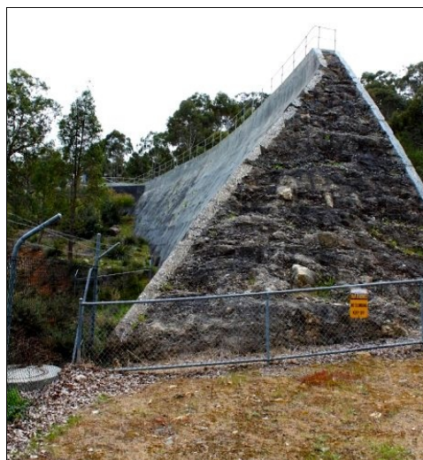
Old Victoria Dam wall cut when a new wall was built 300m upstream in 1990 Photo Stuart Smith
