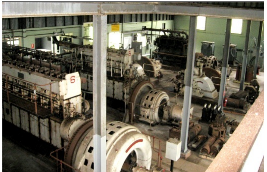
Diesel Engines 5 & 6 with alternators are later additions. The two original turbines are visible beyond generators 5 & 6 to the right. In the back corner, the diesel engine & generator are probably the original Mirrlees engine with its Brush alternator. Photo - Gary Estcourt
