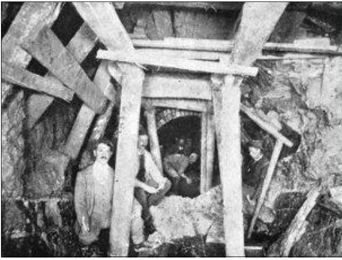
Tunnelling the North Yarra Main Sewer. Image - Water Services Assoc of Aust
