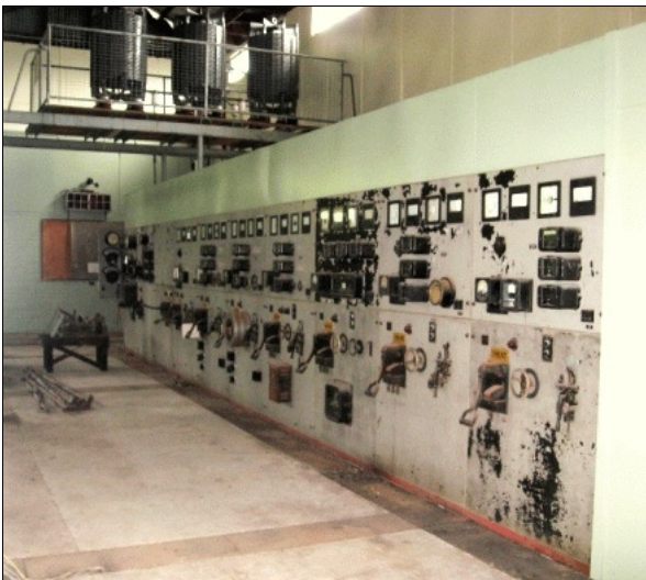
The Hydro PS Switchboard
