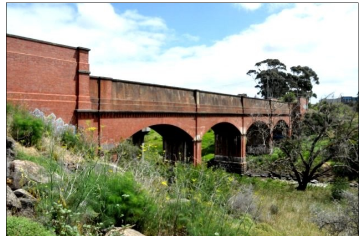
Main Outfall Sewer Aqueduct crossing Kororoit Creek. This aqueduct is now used as a cycleway, from Brooklyn to Werribee. Photo - Owen Peake.
