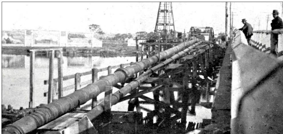
The original 12 inch main & later 21 inch main from Victoria Reservoir cross the Swan River next to the Causeway bridge at Perth. Photo courtesy Water Corporation
