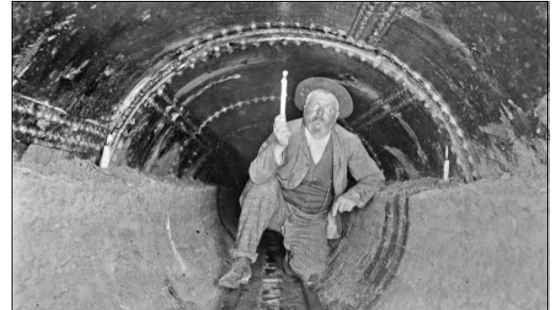
Inspecting the rising main between Spotswood and Brooklyn. Corrosion in this main ultimately led to the closure of Spotswood Pumping Station. The inspector appears to be holding a candle – a dangerous procedure! Image source not known
